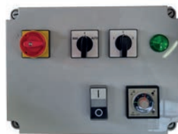
7042 - Panel control with radio remote control
